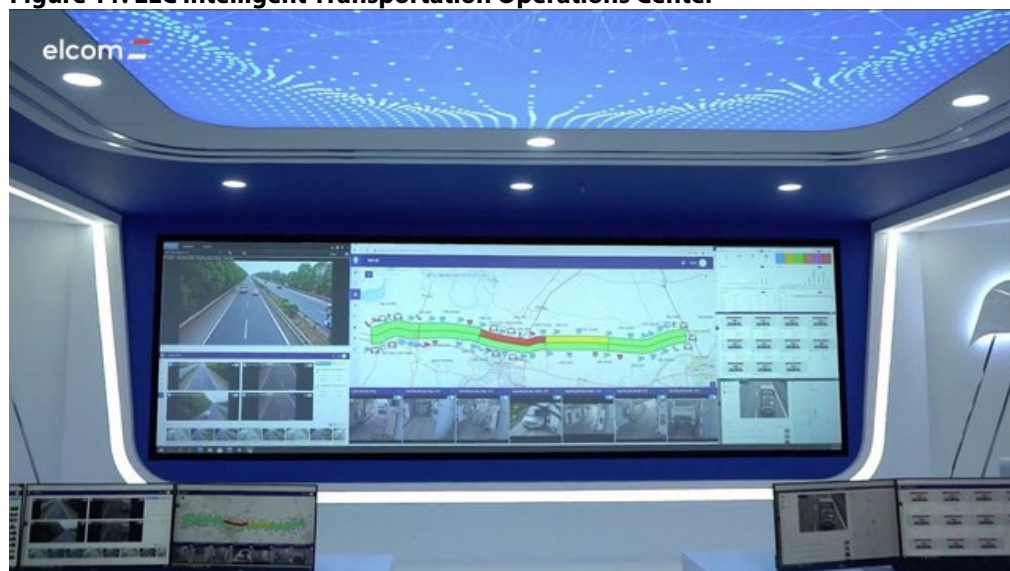
Figure 11: ELC Intelligent Transportation Operations Center
