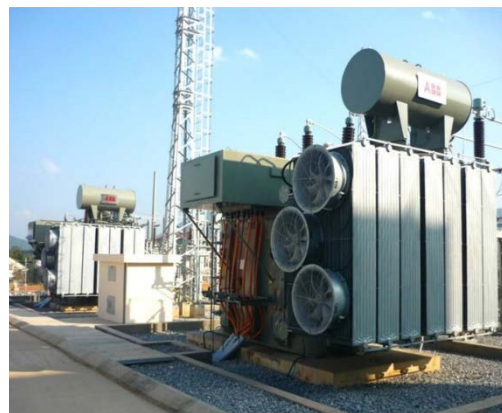
Figure 3: Supper high voltage substation
